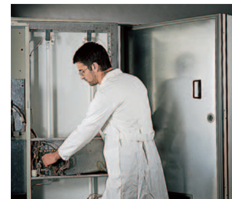
Counterdoor closed on the cabinet during maintenance and programming operations
